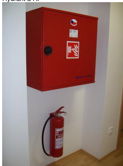
Hydrant a HP
